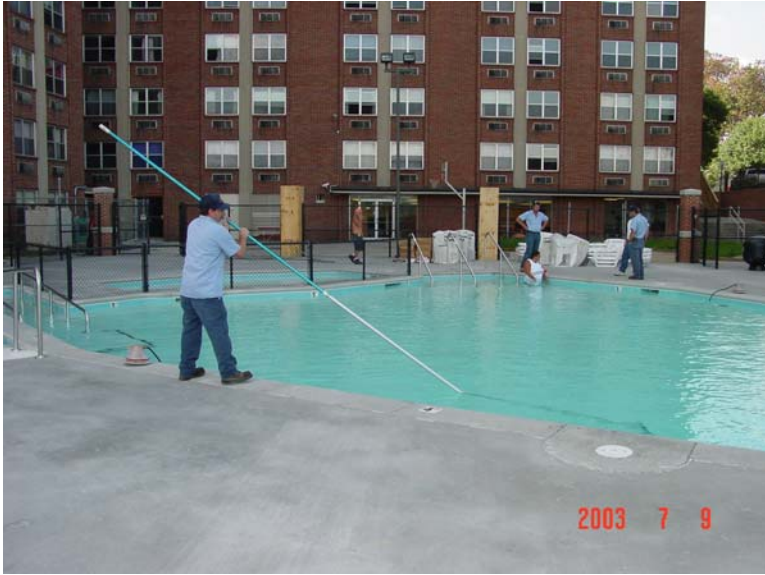
Bryan (Brownie) Shirk puts some finishing touches on the recently completed pool renovation at Laurel Apartments.
