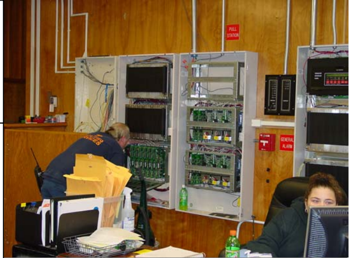
Talk about getting lost in your work. Mike Nelson almost disappears into the fire alarm panel at Hess Hall.
