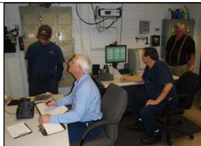
Steam plant employees at work in the control room. The plant is automated and can be run entirely by computer.
