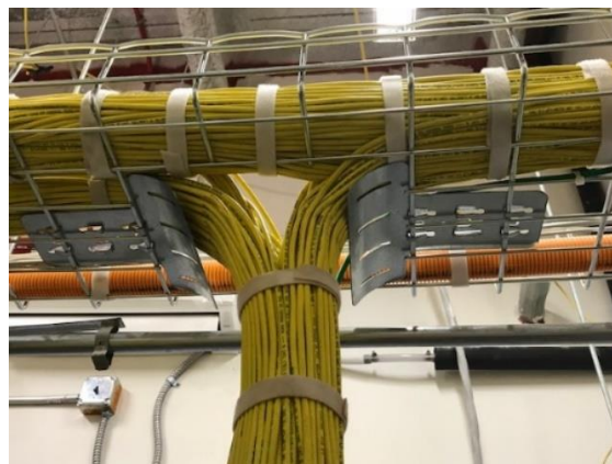
Figure 25: Typical Cable Tray installation
