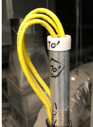
Figure 28: Conduit with Required Bushing
