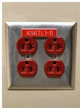
Figure 5: Typical Generator Feed Outlet Identification
