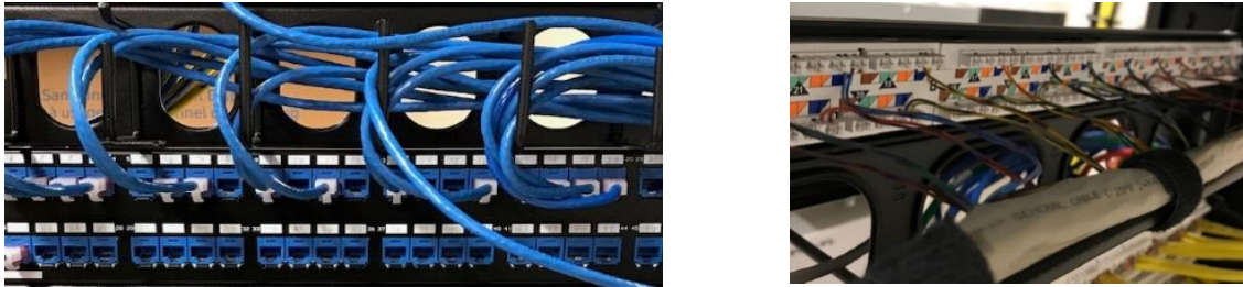
Figure 19: Typical Analog Cabling Deployment
