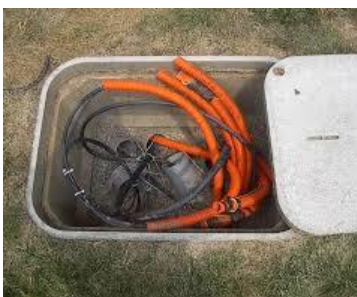
Typical Handhole Box
