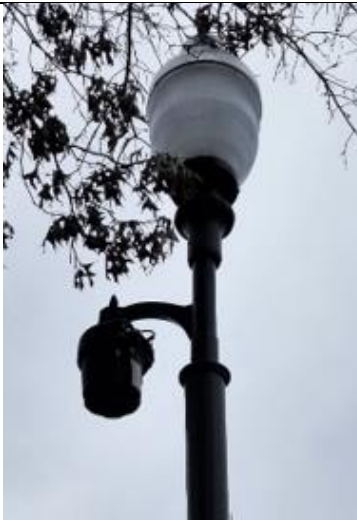
Light Pole with Surveillance Camera and Wireless AP
