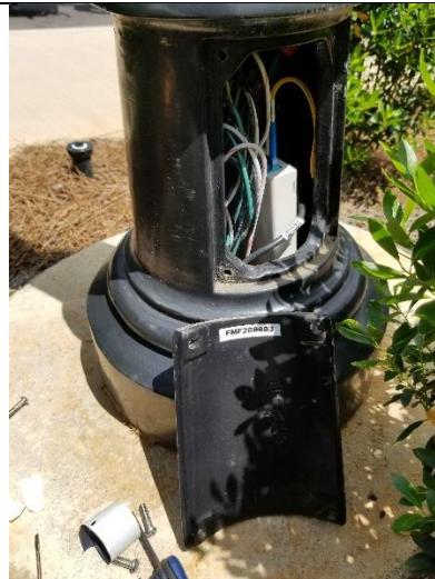
Sample Light Pole Access Panel Labeling
