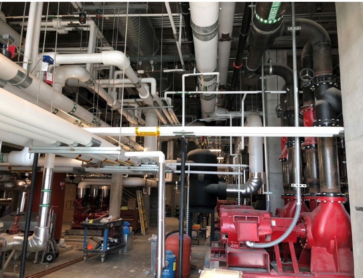
▲ Zeanah Chiller Plant
